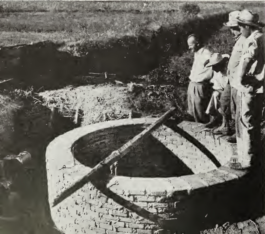
This new irrigation well boasts a motor pump.
